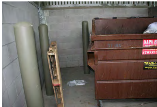
Bollards reduce useable enclosure space and are not permitted inside enclosures.
